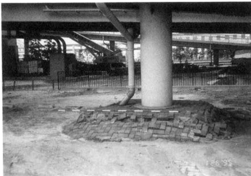
図-5.7 橋梁基礎周辺の液状化 (六甲アイランド北岸) (Settlement of Ground due to Liquefaction near Pier Foundation)
