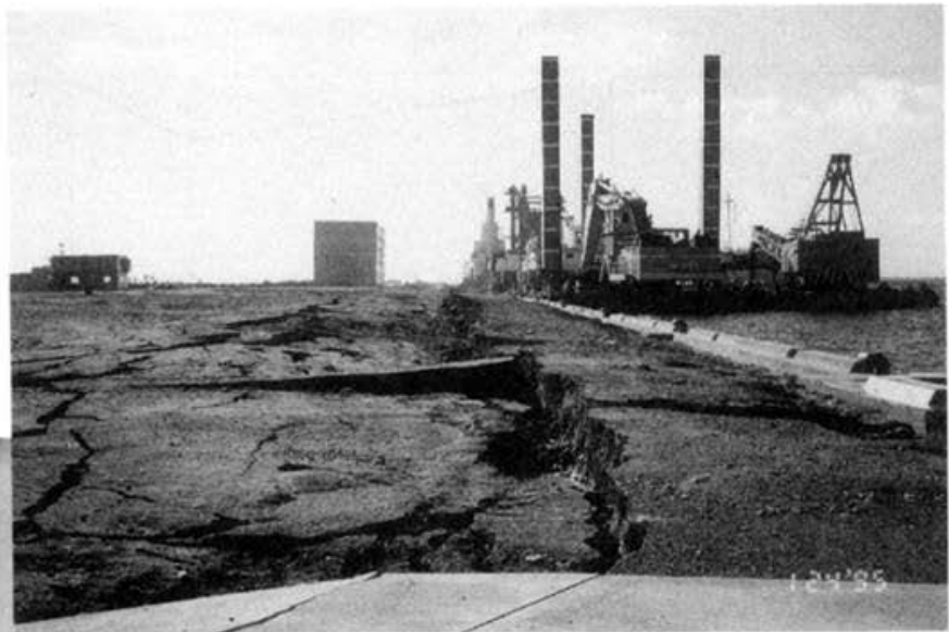
図-5.3 甲子園埋立地護岸の側方流動 (Lateral Movement of Ground near Breakwater)
