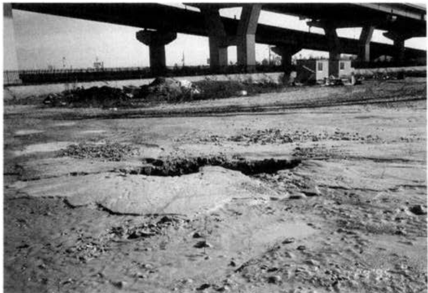
図-5.5 現場近くの地盤の液状化 (Liquefaction of Ground near the Collapse Site)
