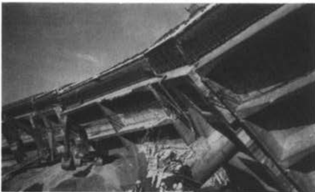
Photo 2.1.5 HANSHIN EXPRESSWAY (Higashinada-Ward - Uozaki-Honmachi)
