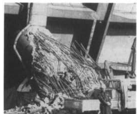
Photo 2.1.6 HANSHIN EXPRESSWAY (Higashinada-Ward - Uozaki-Honmachi)
