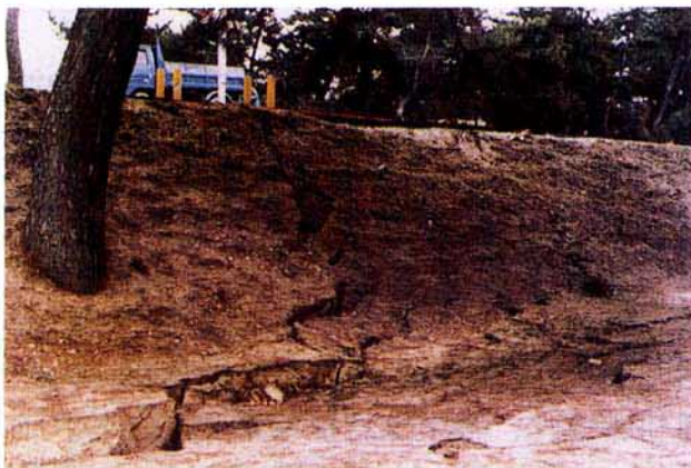
(a) 堤防表のり面の亀裂
