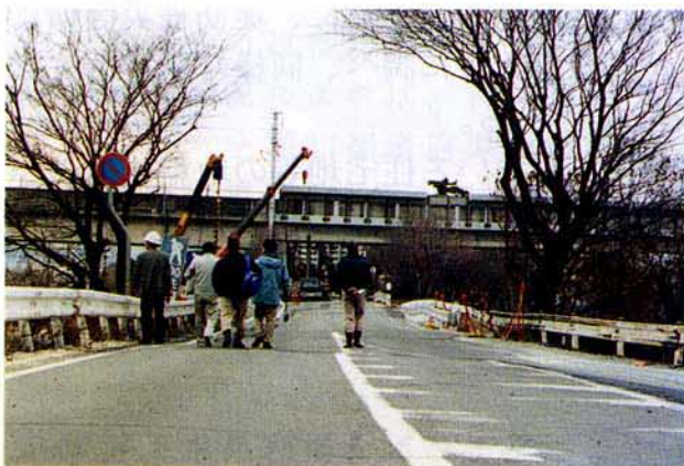
(a) 堤防天端の波打ち
