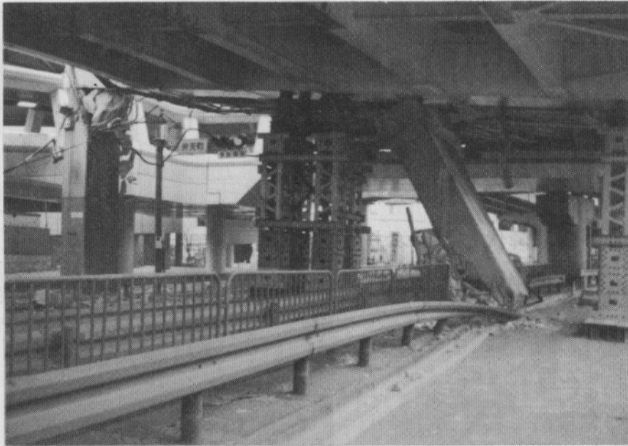
写真 5.6.2-5 中柱のせん断破壊 Photo 5.6.2-5 Shear Failure of a Middle Column
