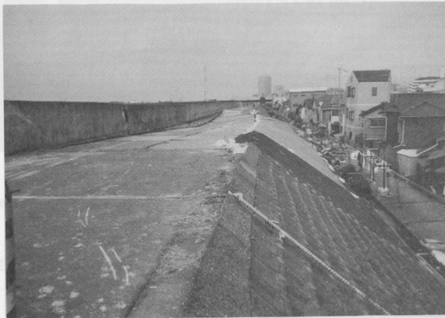
写真-5.8-3 堤体の沈下と裏のりのはらみだし Photo. 5.8-3 Settlement of Embankment and swell of back side slope
