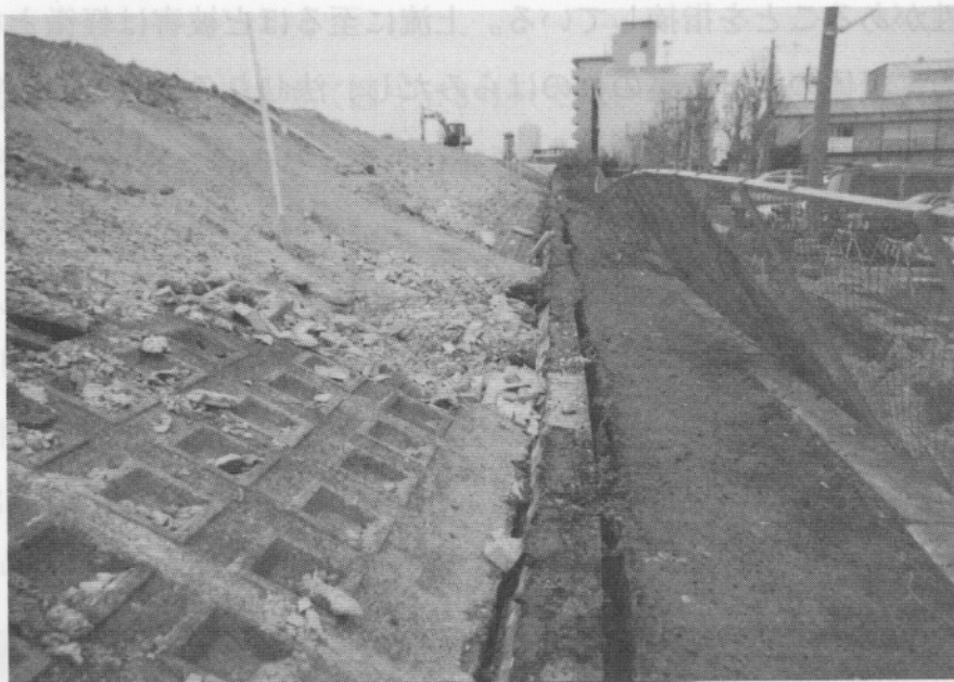
写真-5.8-2 裏のり被覆工の被害とのり尻の亀裂 Photo. 5.8-2 Damage at Back Side Slope Coverage and Crack at Top of Slope
