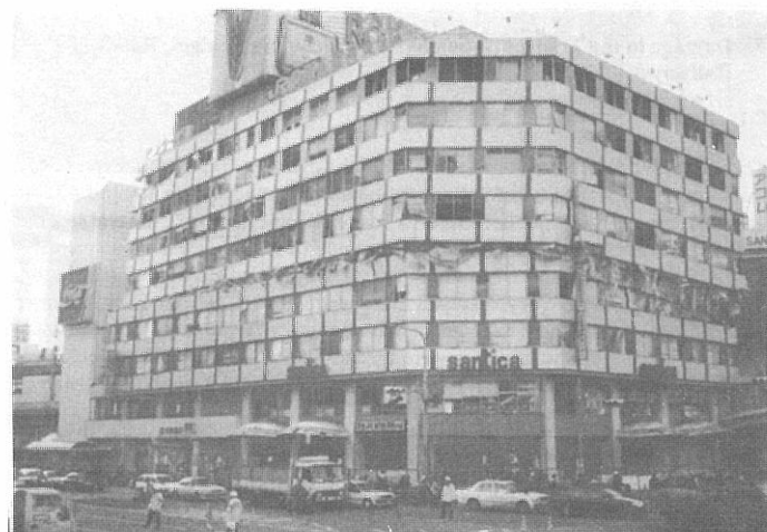
Photo 8 Collapse of the 5th floor of Sannomiya traffic center building
