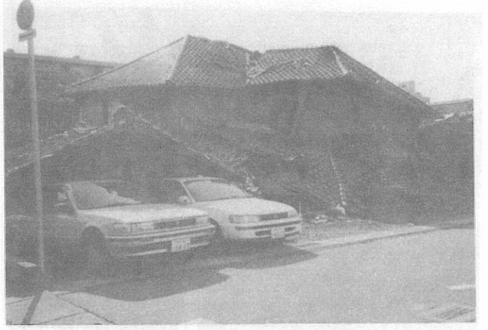
Photo 5 Collapse of timber houses with heavy roof tiles
