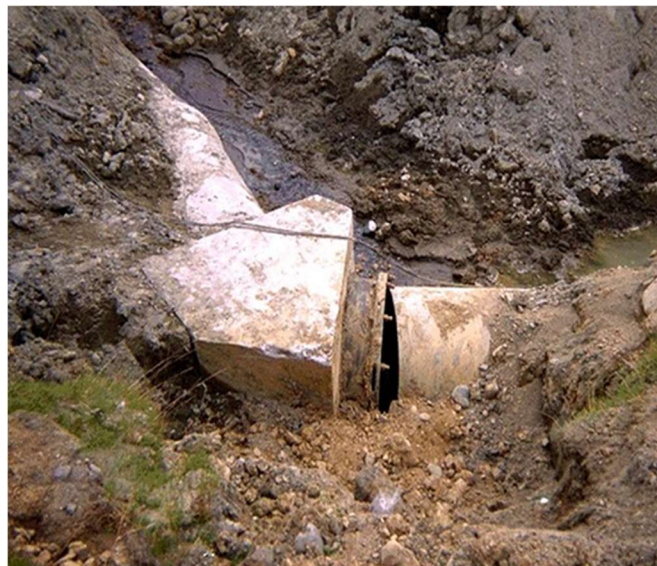
Fig. 1-3 Joint separation due to the 1993 Hokkaido-Nansei-Oki Earthquake (Mohri et al., 1995)
