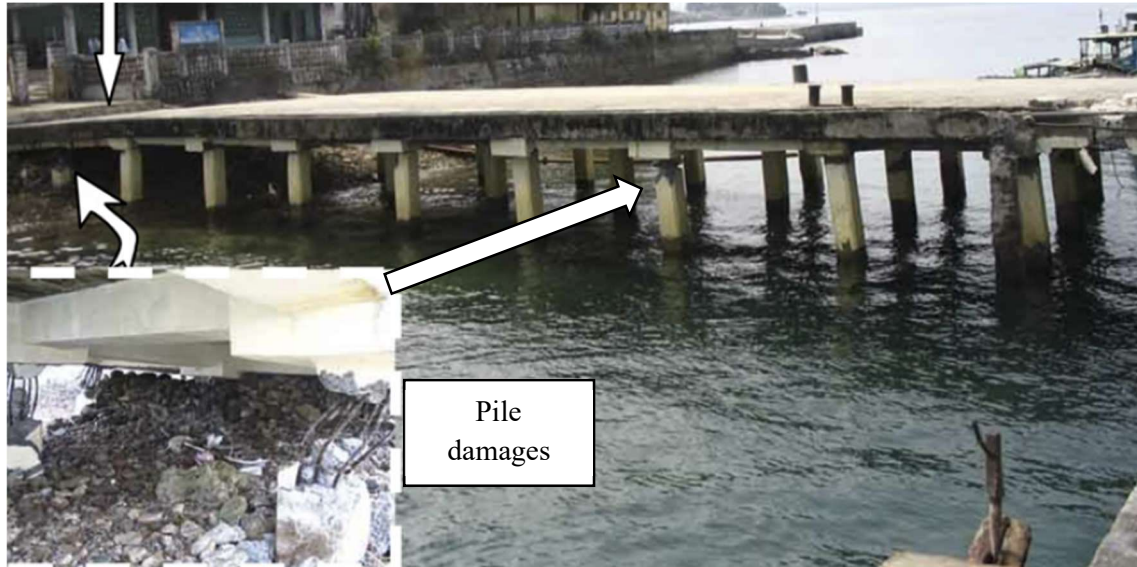
Figure 1.1 The pile damaged in a PSW in Andaman Island
