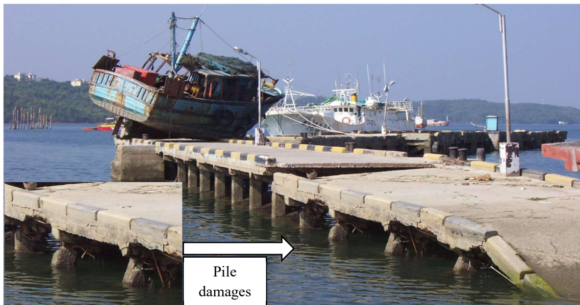
Figure 1.2 The pile damaged in a PSW in Indonesia
