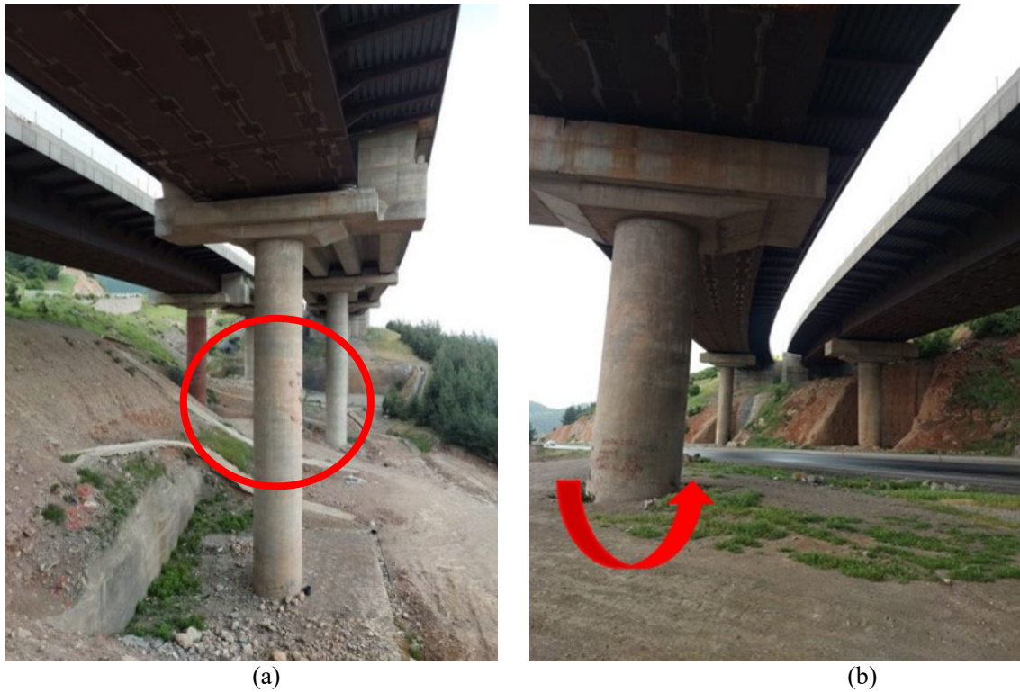
Figure 7 Plastic hinge formation and temporary repair of column and settlement and rotation of the column
