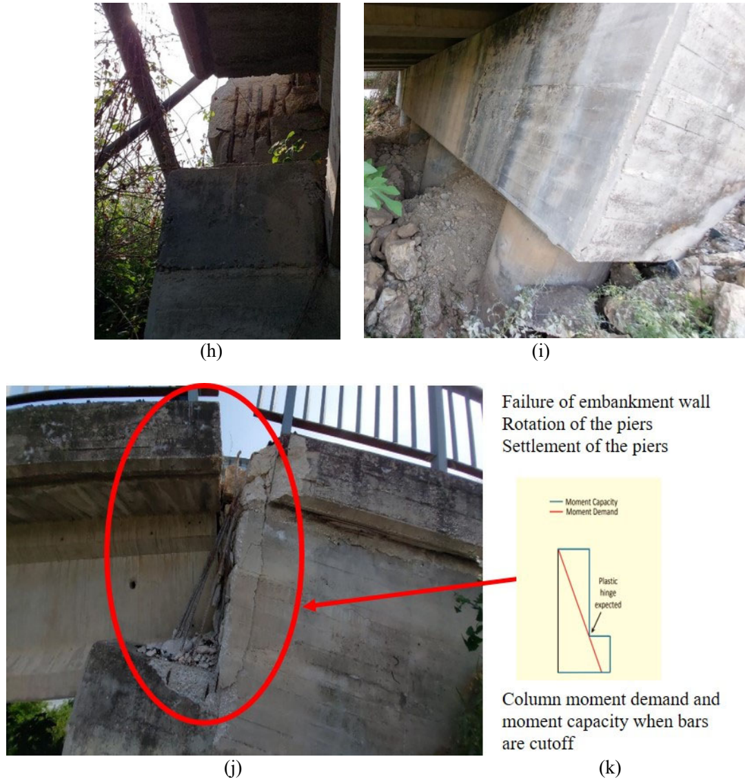
Figure 16 Damages in the bridge Demirköprü, Antakya; (h)insufficient cover of the concrete and corrosion of the rebars (i) failure of embankment wall including rotation of the piers (j) pullouts of the reinforcements and failure of concrete (k) column moment demand and moment capacity when bars are cut off
