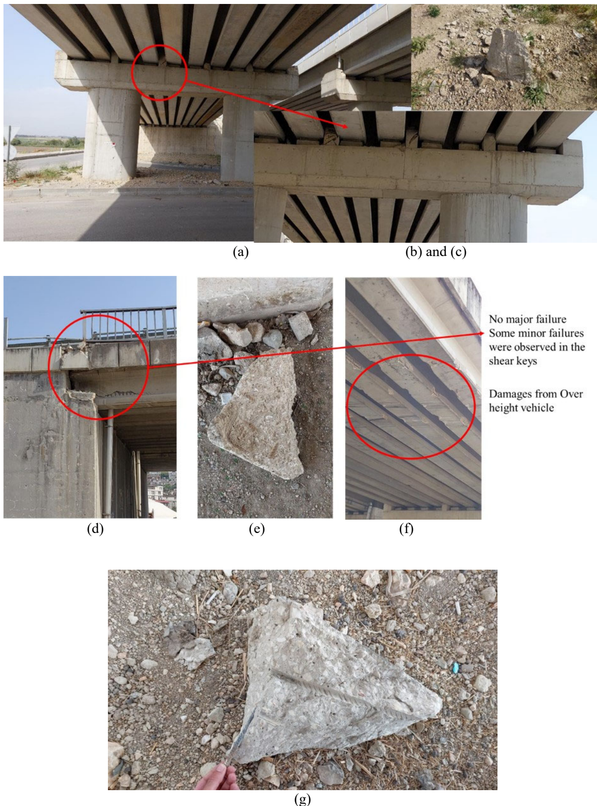
Figure 17 Viaduct in Antakya city; (a) and (b) failure of shear keys (c) falling off concrete segments (d) shear key failure and shear crack formation in the deck (e) segment falling (f) damages by over height vehicles (g) rebar pullout and insufficient effective length
