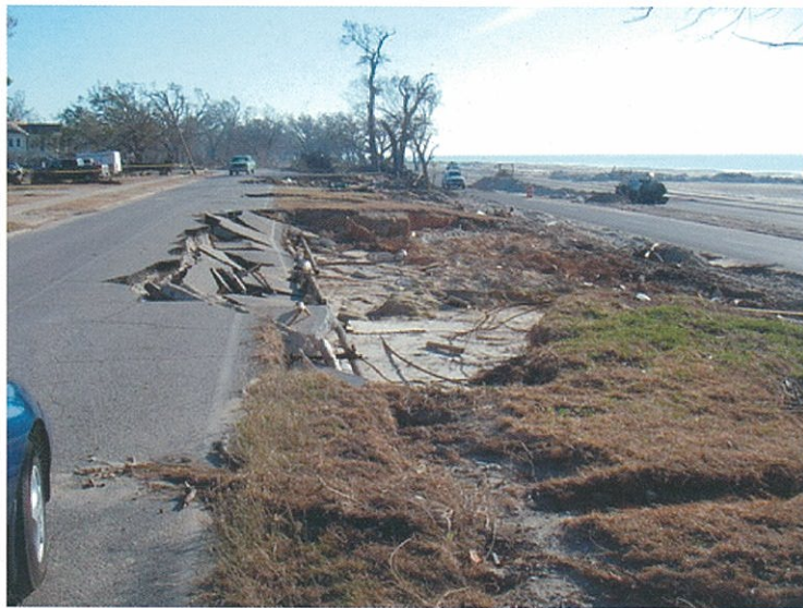
Photo #28. Pass Christian, MS. Road on a coastal bluff, washed away by the surge.
