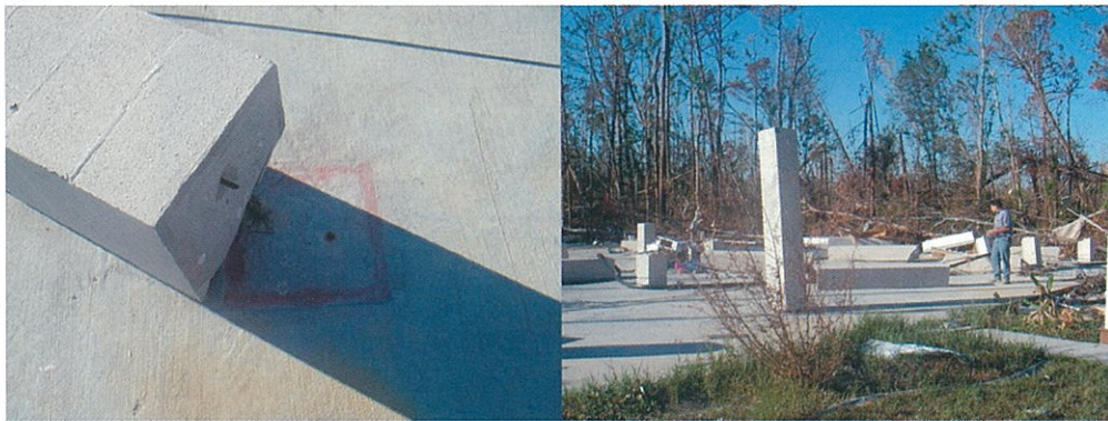
Photo #20. Diamondhead, MS. Pilings from atop which a home had been carried away by the surge. These concrete piles, very weakly attached to the foundation below them (by only a single piece of rebar), toppled.
