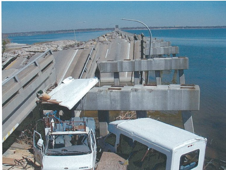
Photo #38. US Highway 90 bridge over Biloxi Bay. Decks were pushed off their piles by surge and waves.
