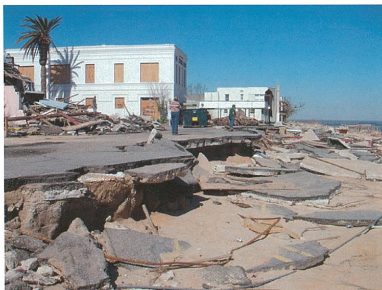
Photo #15. Bay St. Louis, MS. Coastal road and buildings destroyed by the surge.
