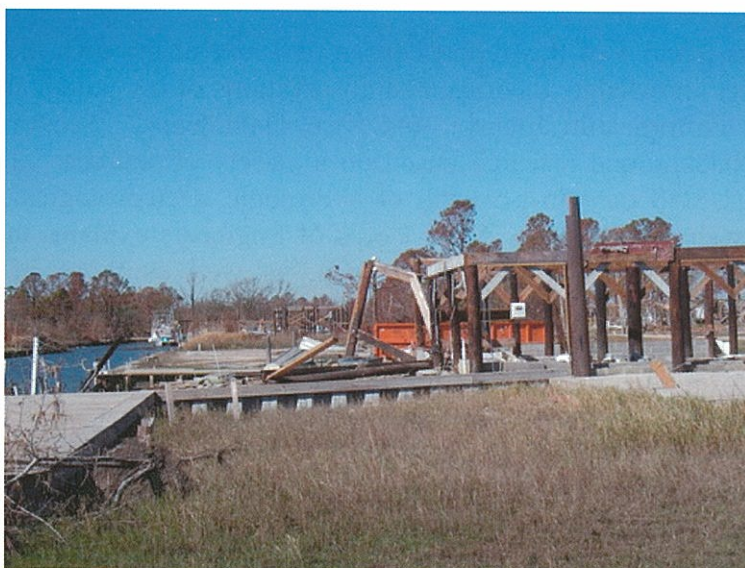
Photo #3. South of Pearlington, MS. Piles that had supported homes, which floated away (landward) in the surge. The bayou off which the surge entered the region is visible on the left.
