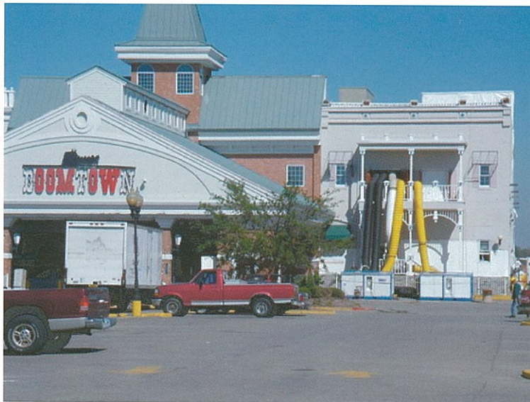
Photo #35. Biloxi, MS. Casino with dehumidifying ducts running out of its 2 nd story windows, in an attempt to clear the place of mold.
