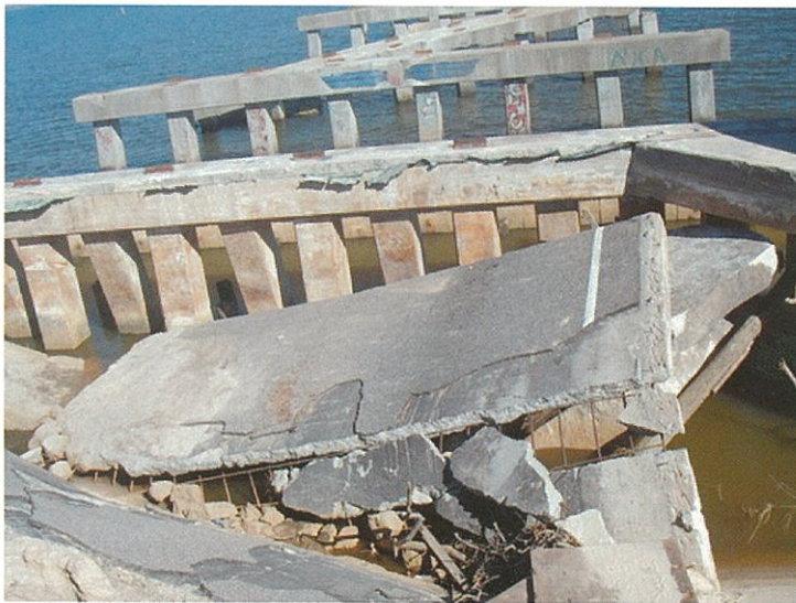
Photo #18. The US Highway 90 bridge over St. Louis Bay, MS. Decks were pushed off their piles by the surge and waves.
