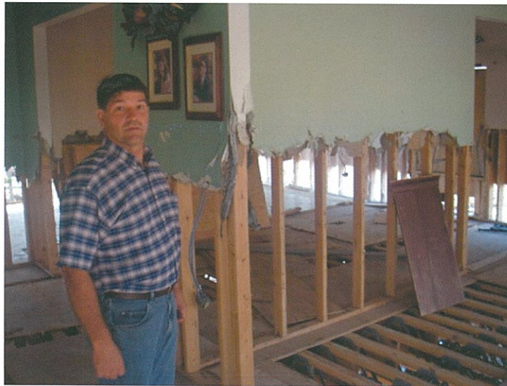
Photo #22. Diamondhead, MS. 2 nd floor of a flooded home. All soft materials were destroyed.
