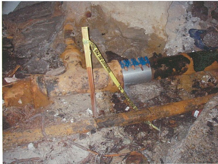
Photo #25. Pass Christian, MS. Water and gas pipelines under a road which had been washed out in the surge. The steel sleeve on the water main is a temporary repair, to allow the system to be repressurized.
