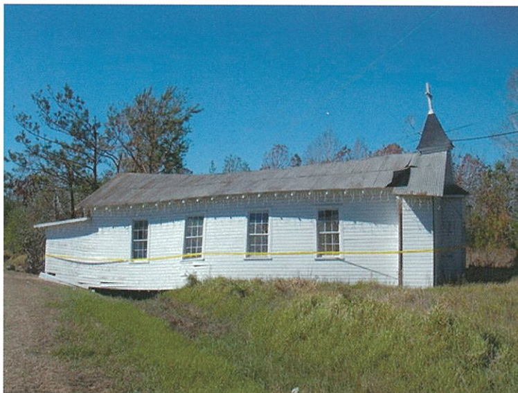
Photo #4. South of Pearlington, MS. A church which had floated off its foundation during the surge, and landed in this spot when the floodwaters receded. Spray painted on the siding on the left-hand side of the photo are the words "Do not destroy. Historical building. Built 1868 by C LaFontaine."
