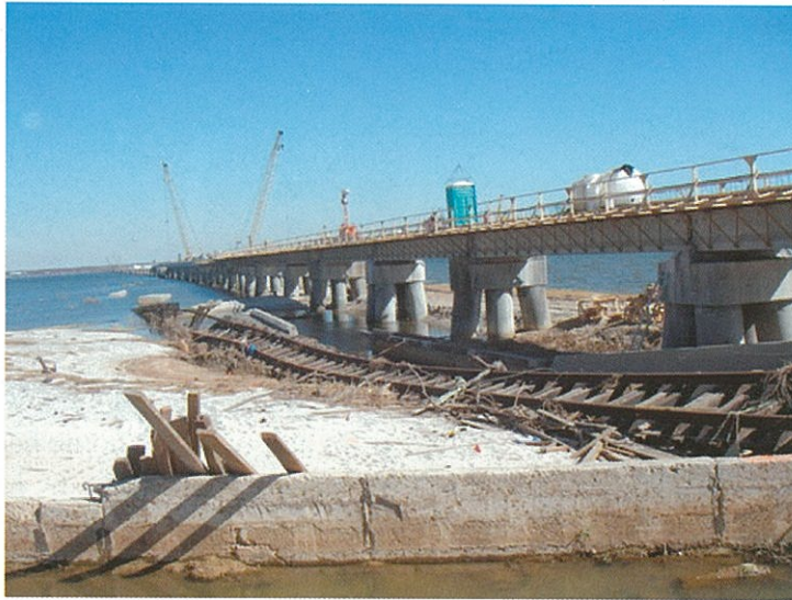
Photo #17. Railway bridge across St. Louis Bay, destroyed by the surge, and now under repair from both directions.
