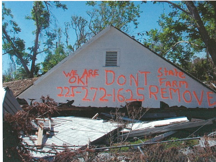
Photo #13. Waveland, MS. Roof sitting atop a wrecked home.
