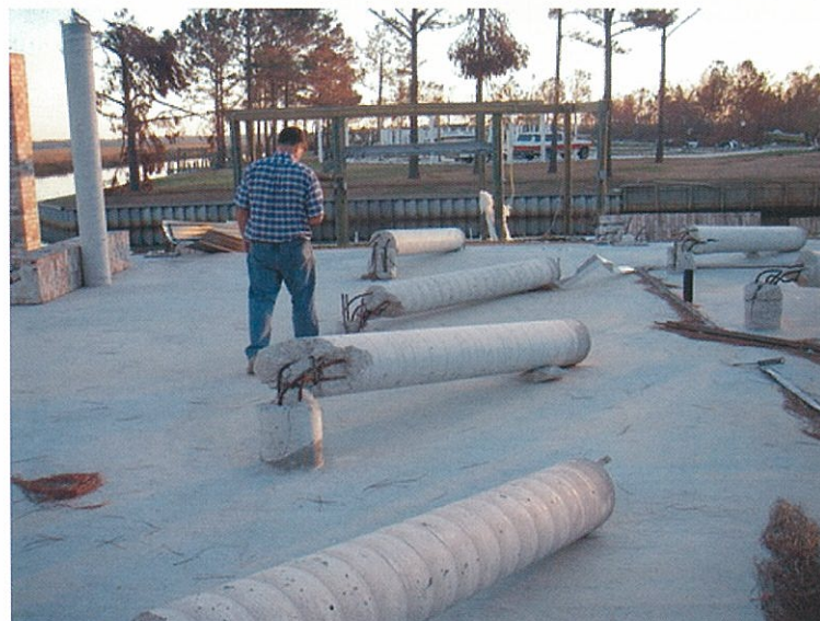
Photo #21. Diamondhead, MS. Piles from atop which a home had been carried away by the surge. These concrete piles, though fixed strongly to the foundation by pouring the foundation around the piles, as well as by running many pieces of rebar from the foundation to the piles, failed.
