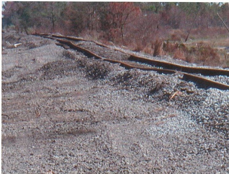
Photo #2. South of Pearlington, MS. Railway damaged by the surge and associated debris, and gravel ballast scoured seaward by the surge.
