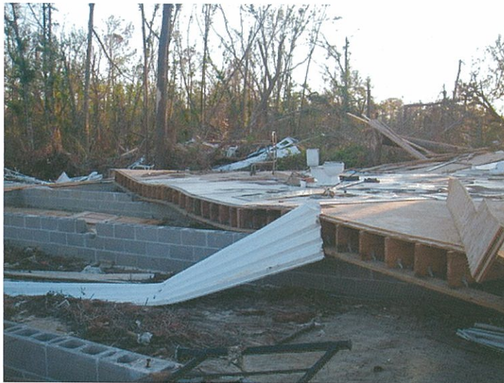
Photo #23. Diamondhead, MS. Floor of a home which had floated off its foundation blocks in the surge.
