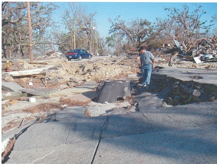
Photo #29. Pass Christian, MS. Manhole intact despite the road around it having been destroyed by the surge.
