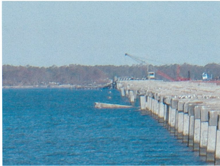
Photo #19. Piles supporting the US Highway 90 bridge over St. Louis Bay, MS. Some piles failed in the strong tidal currents induced by the surge.
