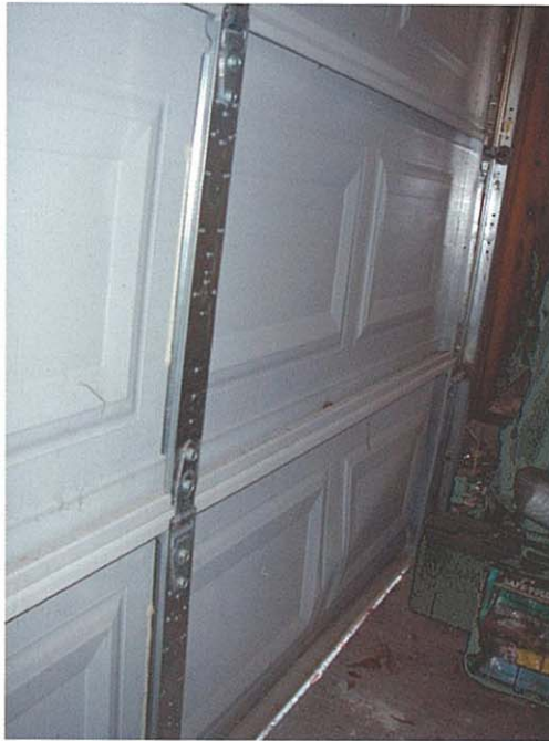
Photo #41. Slidell, LA. Garage door of a home, with its bottom panel buckled and seal broken by surge waters.
