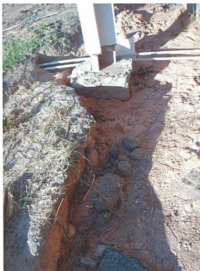
Photo #27. Pass Christian, MS. Earth scoured away from around a building's pile by the surge.
