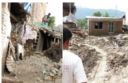
Photo. 3. Ready to fall buildings and streets still to be cleared even after six months (Sept, 2015)
