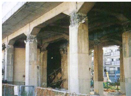
(b) Flexure failure of a viaduct
