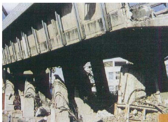
(a) Shear failure of a viaduct
