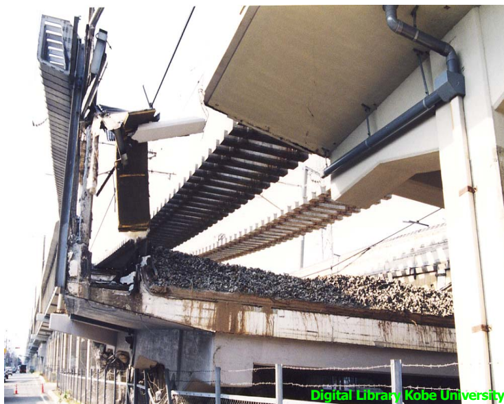
Cave-in of viaducts in Kobe earthquake
