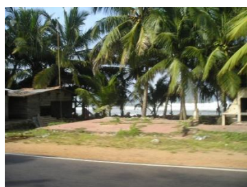
① Totally damaged permanent house at Hikkaduwa-2006
