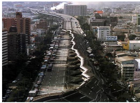
Damage for Infrastructure
