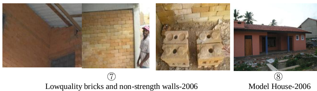
Fig.3.35: Construction Failures and Experimental Model House on 2006
