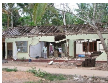
Partially damage (unusable) permanent house
