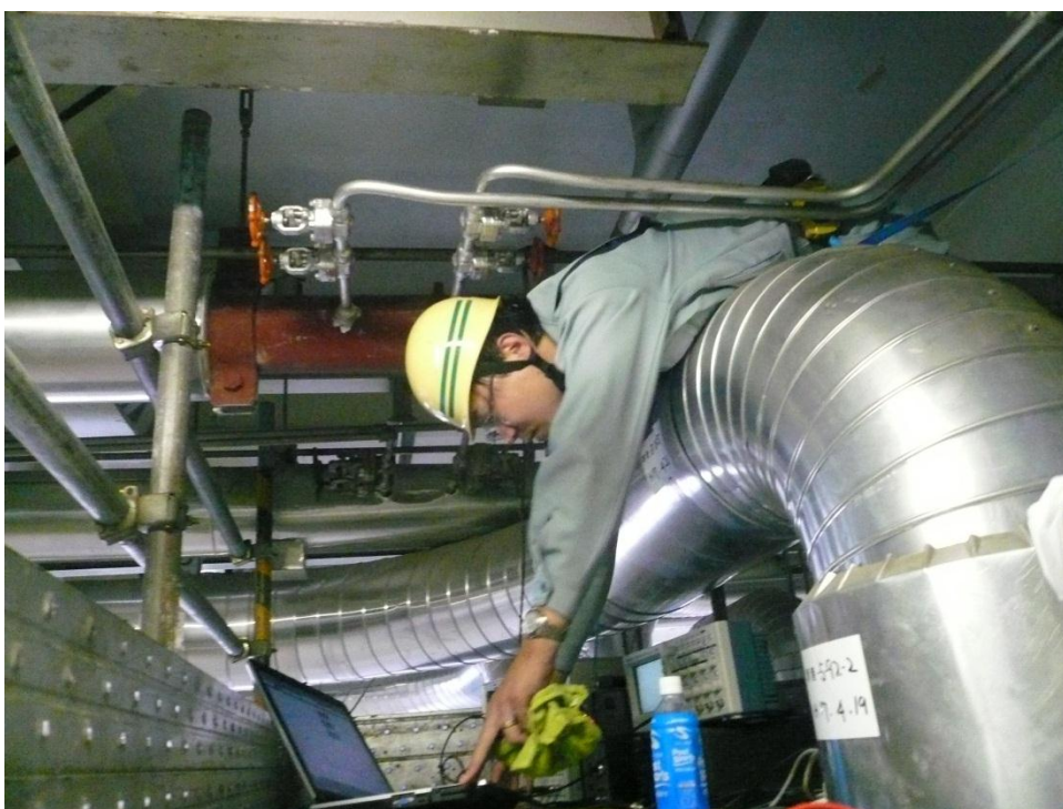
Fig. 5.3.2-4: Measurement field in thermal power plant
