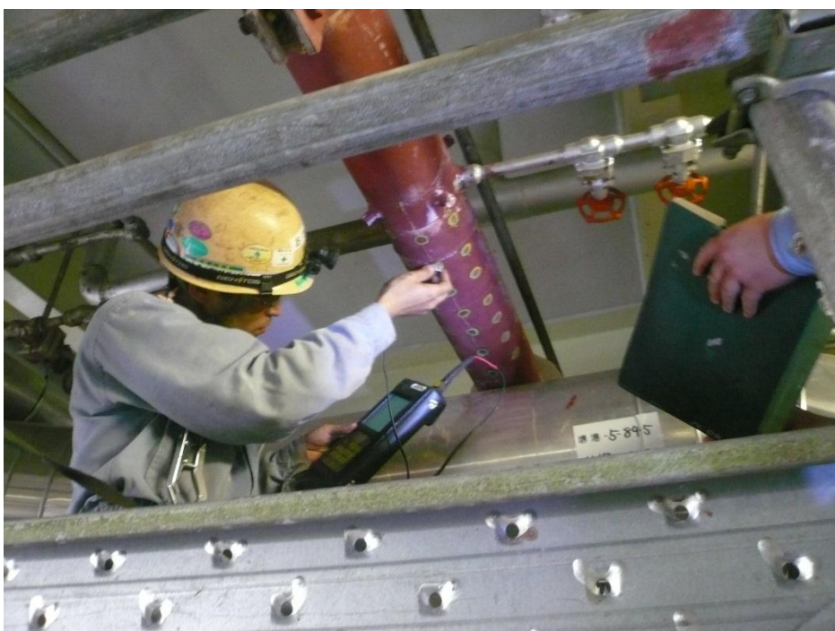
Fig. 1.2.1-6: Thickness measurement work using UT. Measurements are performed by two workers. Main worker measures wall thickness. Another worker records measurement results.
