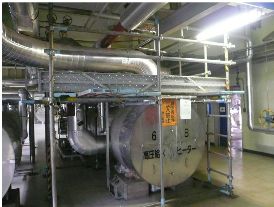
Fig. 1.2.1-4: Scaffolding for thickness measurement. Scaffolding must be made, when work location is a high place.
