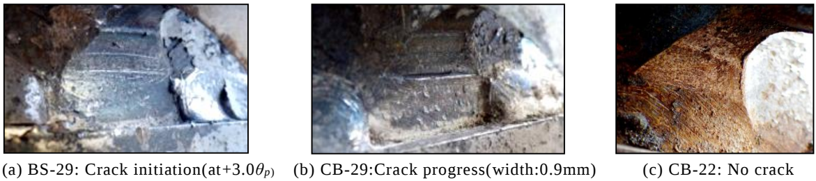
Fig. 2.10 Typical crack initiation and progress at the root of scallop in the first cycle of +4.0\theta_p
