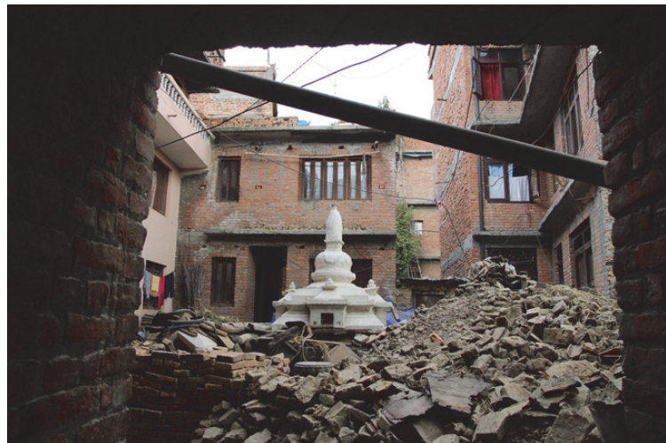
Figure 26 Damaged buildings with the Chowk , in Sankhu. This Chowk was changed by rebuilt. (photo by T. Ohsumi, taken after earthquake in Sankhu)
