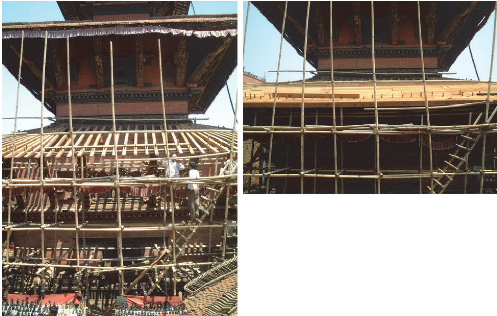
Figure 30 Renovation of a temple's roof was carried out in 2015 (photo by T. Ohsumi).
