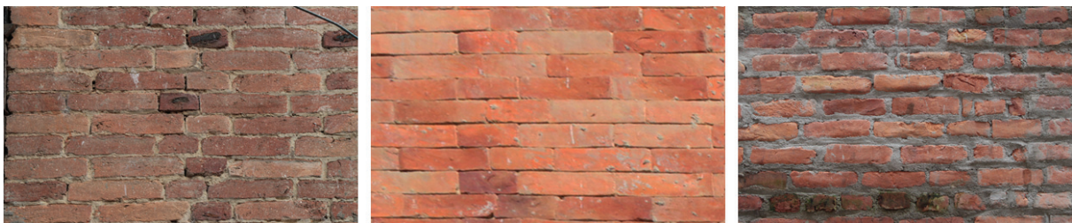
Figure 4 Comparison of brick with different kind of mortar as BM, BMW, BC.
