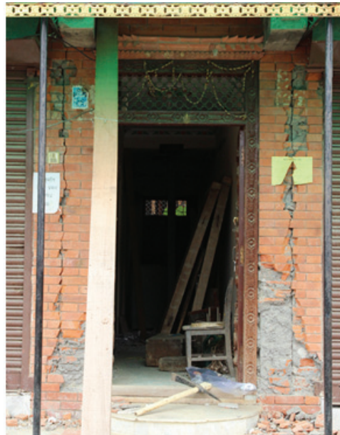
Figure 7 Entrance damage, damage level was deemed to be “yellow”. (photo by T. Ohsumi)
