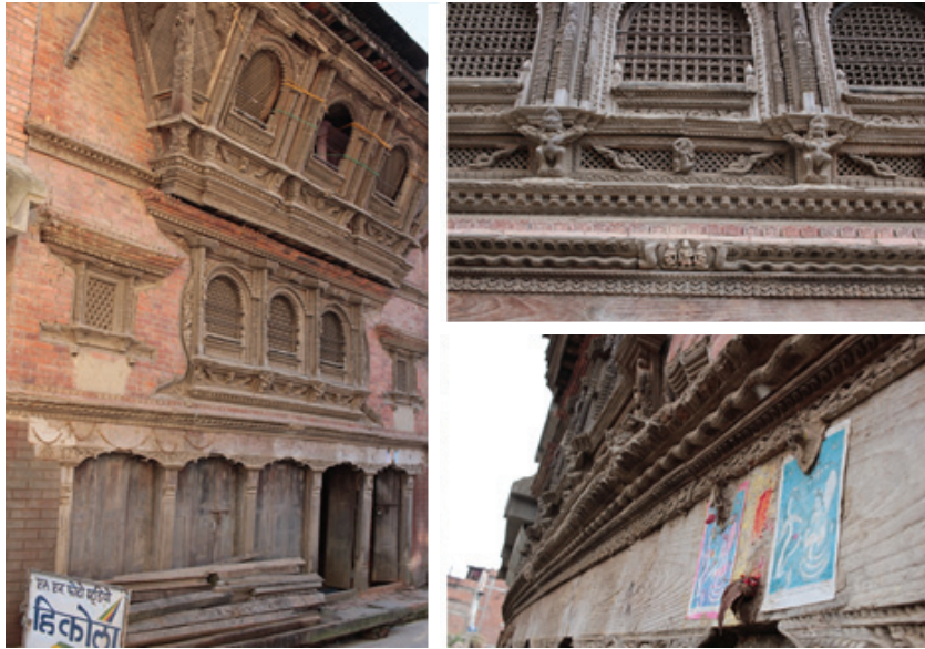
Figure1 Building constructed over 100 years ago that was slightly damaged by the Gorkha earthquake. The building has a snake (Naga) band surrounding it between the first and second floors. (photo by T. Ohsumi, taken after the Gorkha Earthquake in Sankhu)
