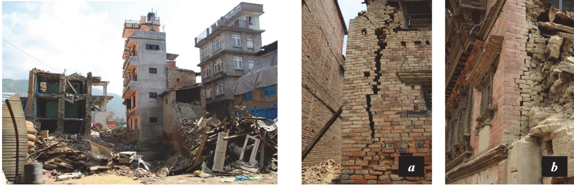
Figure 20 The damage to RC structures was generally minor. These structures were mainly five to six story buildings. Many of the non-engineered masonry structures that experienced complete collapse or partial damage were two to four story buildings in Sankhu ( left ). Damage in non-engineered masonry structures was initiated by vertical cracks in the corners of the buildings ( a ), which contained no RC columns ( b ). (photo by T. Ohsumi).
