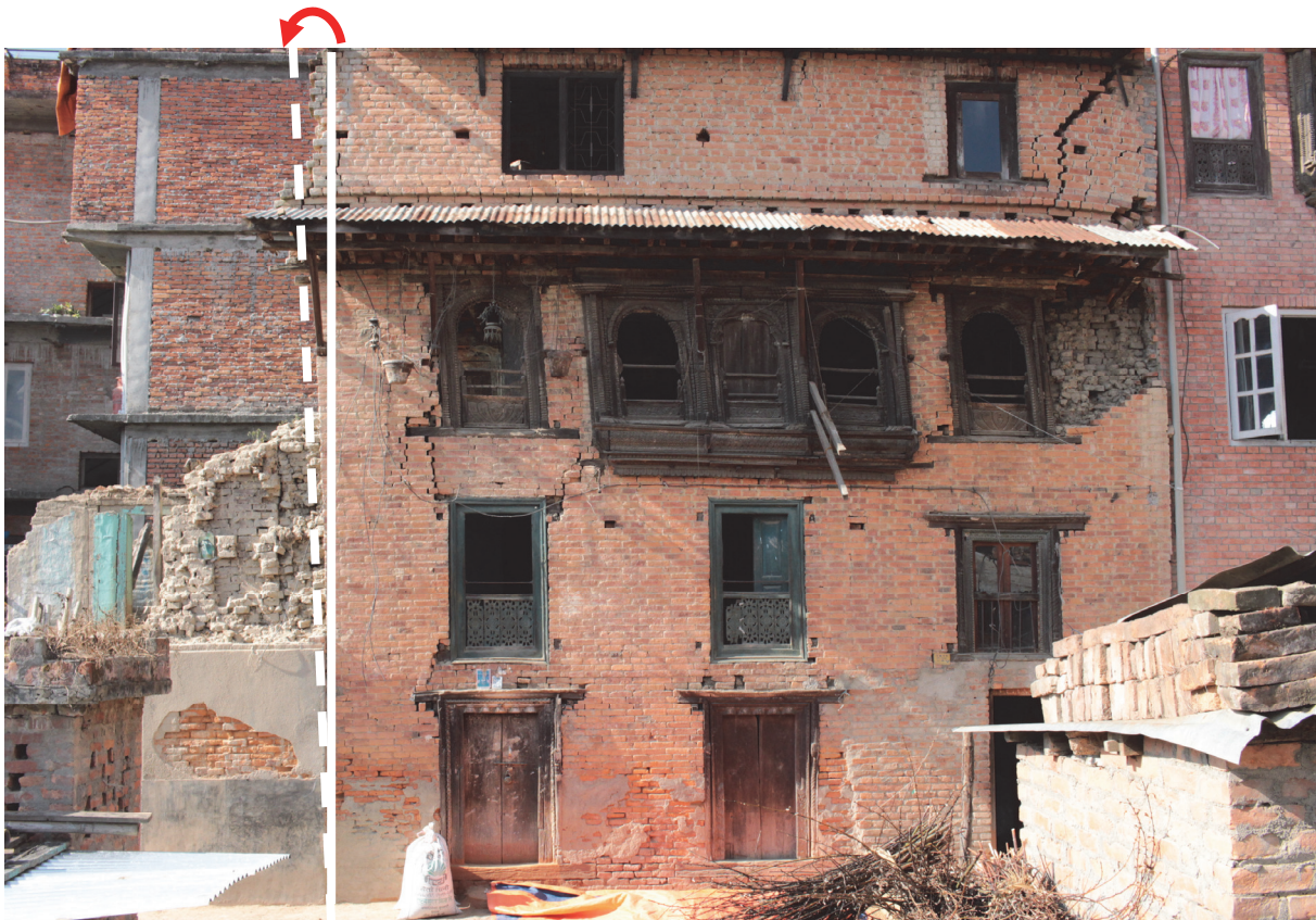
Figure 11 Traditional structures caused residual deformations and defective corners of the building related to the 2015 Gorkha Earthquake in Khokana (photo by T. Ohsumi after the 2015 Earthquake).
