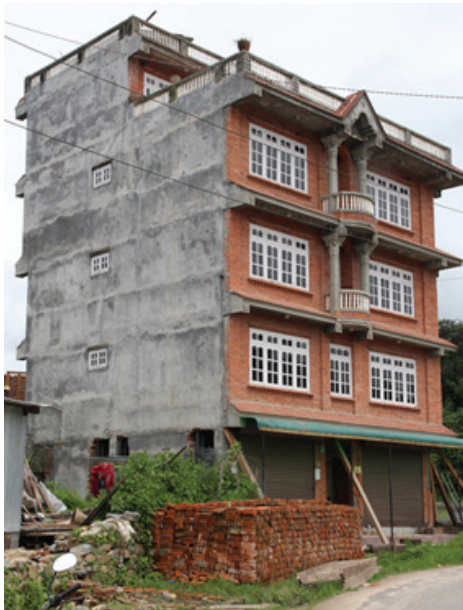
Figure 6 Damaged housing in Sankhu. (photo by T. Ohsumi)
