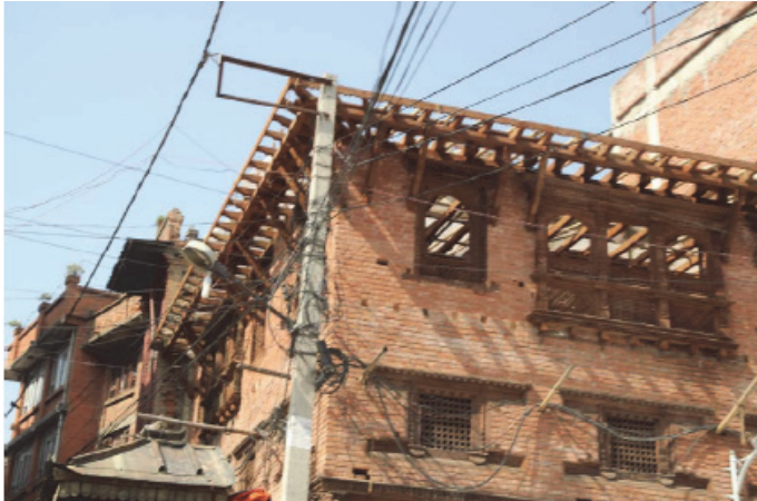
Figure 31 Renovation of a house roof was carried out in 2015 (photo by T. Ohsumi).
