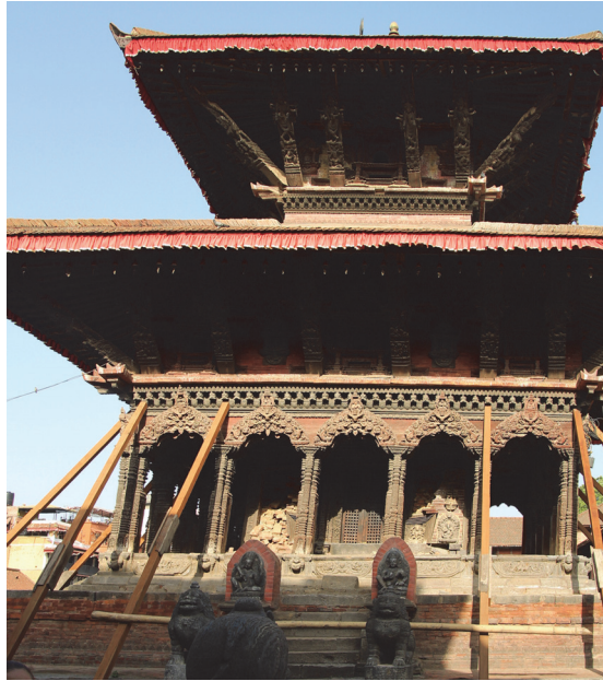
Figure 12 Temple caused residual deformations and defective corners of the temple related to the 2015 Gorkha Earthquake in Patan (photo by T.Ohsumi after the 2015 Earthquake).
