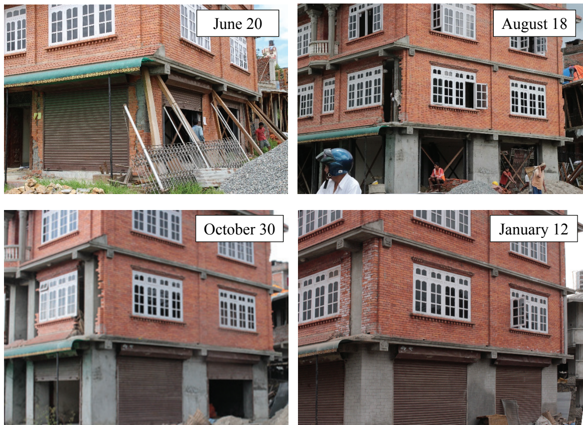
Figure 8 Progress of earthquake repair to a ground floor column. (photo by T. Ohsumi)
