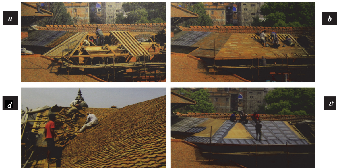
Figure 14 Renovation of the structure and the cover of the roof was carried out in 2011. a : top left Installation of timber rafters, b : hand wood planking, c : waterproof membrane, d : traditional terracotta roof tiles on a mud-bed (from Information plate of Patan Museum).
