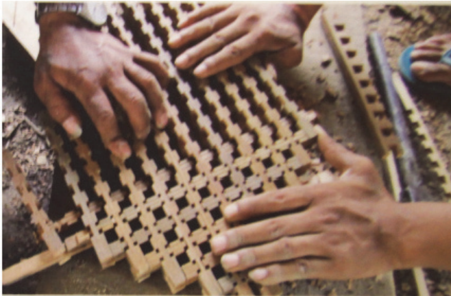
Figure 10 Timber lattice replacements. New timber latticework has been fabricated to replace damaged or lost elements (from information plate at the Patan Museum).
