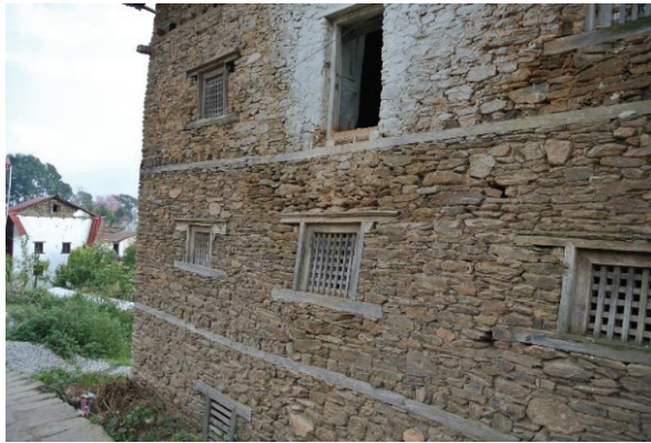
Figure 4 Timber band installed between the first and second floors in a house in Charikot
