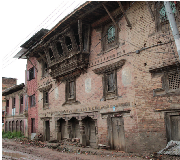
Figure 2 Building that was over 100 years old, showing little damage. (photo by T. Ohsumi, taken after the Gorkha Earthquake in Sankhu)
