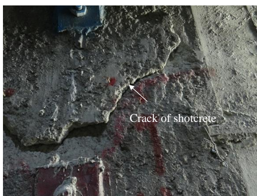
Figure 3.12 Cracking of the shotcrete
