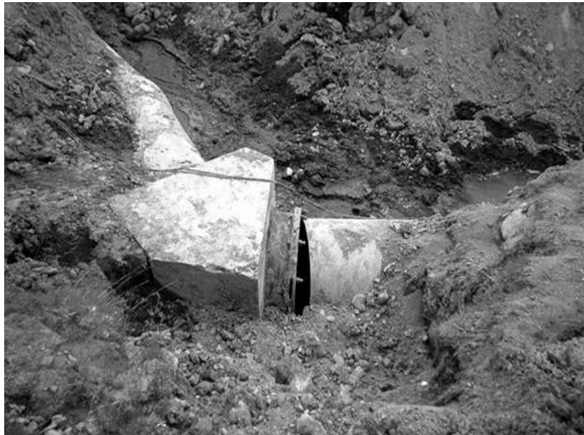
Figure 1.2 Detachment of pipe bend by the 1993 Southwest-off Hokkaido Earthquake (Mohri et al., 1995)
