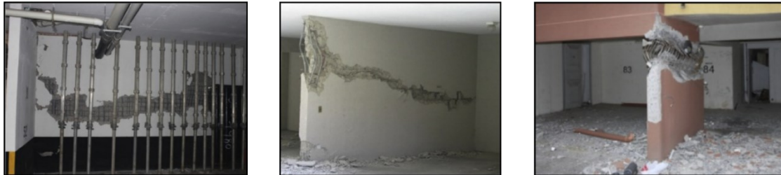
Fig. 1-1 Damaged ductile concrete walls during Chile earthquake [1.2]
